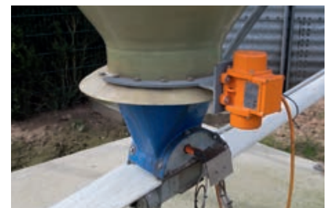
Silo with electric vibrator
