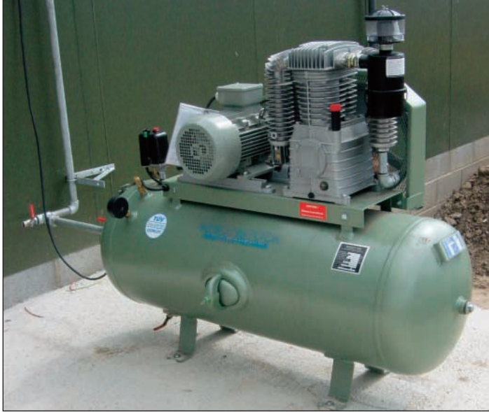
Compressor for the generation of compressed air
